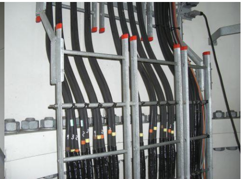
Wind Turbine Tower Internal Piping
