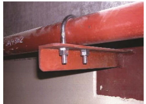
Piping in Power Plant
