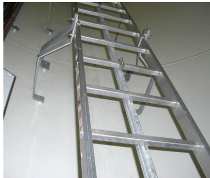
Ladder in Wind Turbine Tower
